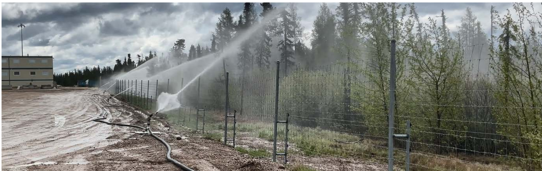
▲ A sprinkler protection system is used at Wolf's Den Camp at Foster Creek to wet down surrounding areas.
